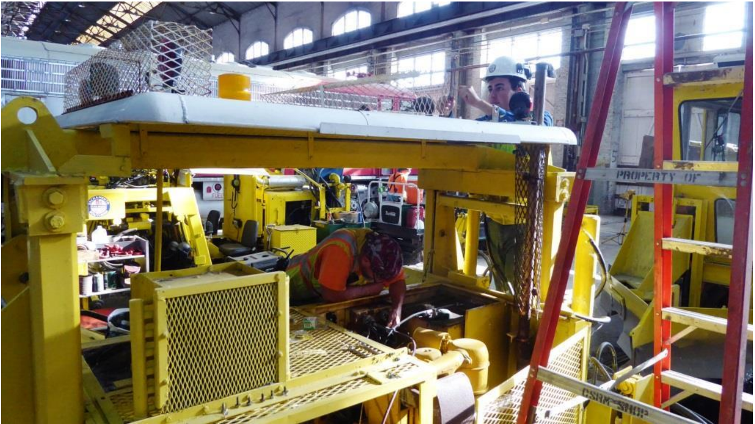
Joe re-works the electrics and Weston installs a horn on the Jackson 125 tie-exchanger
