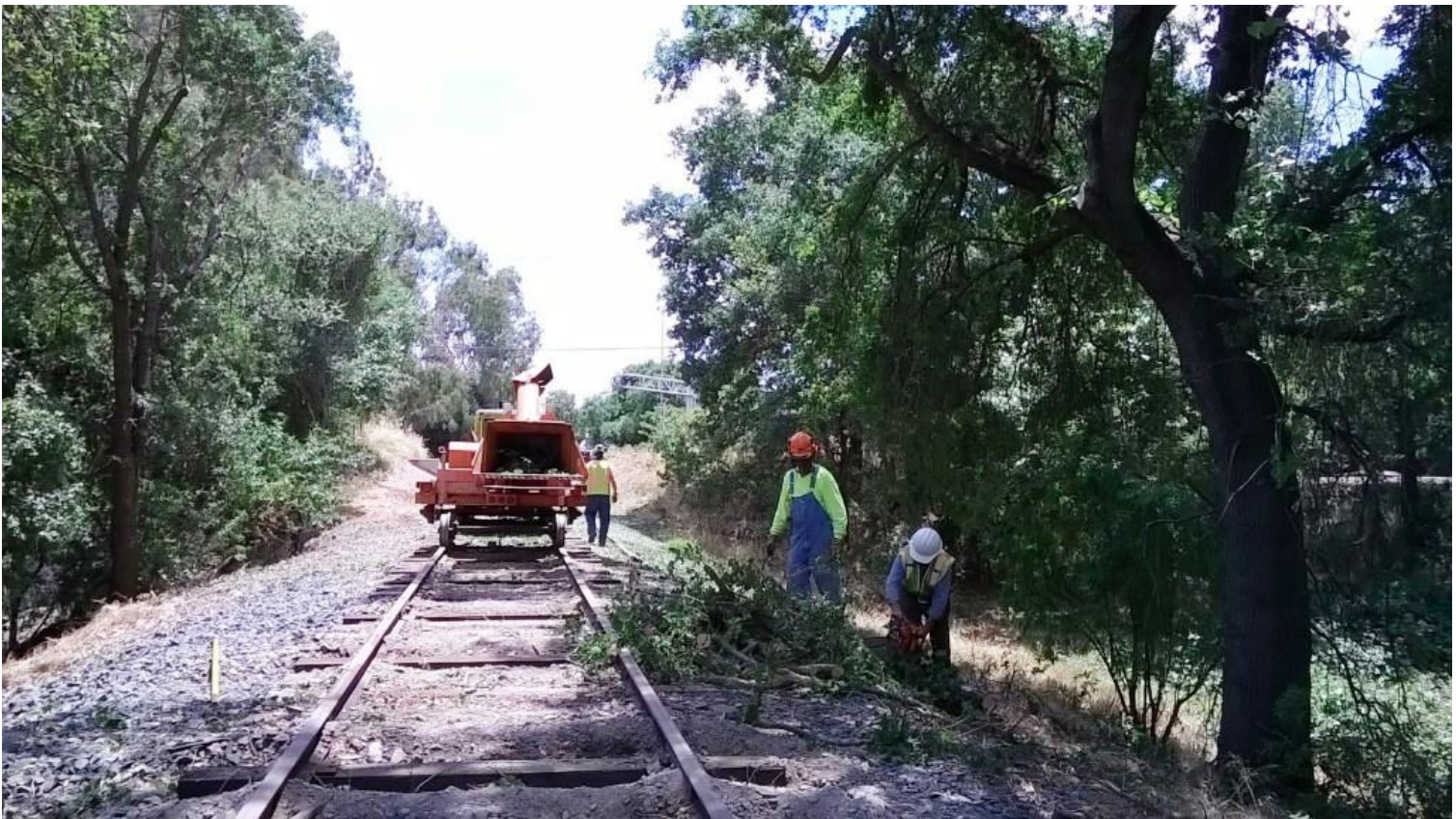
Dave and Mike reducing the green debris to a manageable size to fit into the chipper
